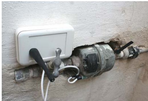
Figure 4: A ZigBee AMR Transponder Latched onto a Water Meter
